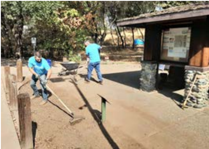
Opening up the kiosk area to the parking lot to create a new entrance.
